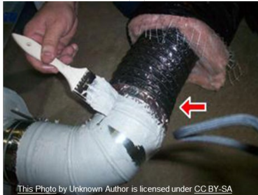
Figure 7: Example of duct sealing
