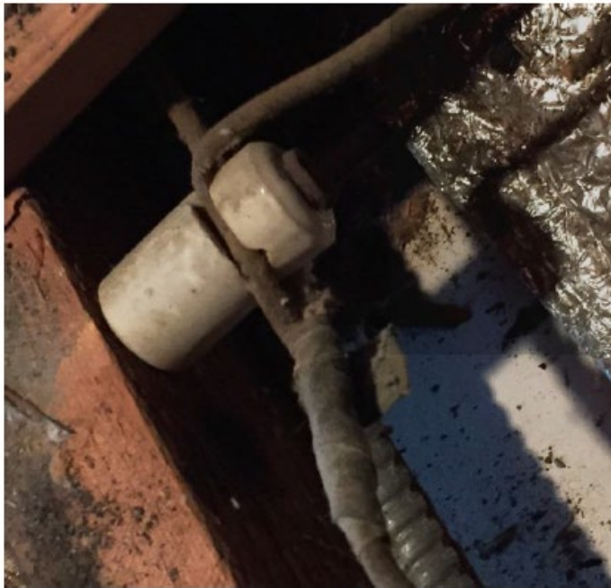
Close-up of typical ceramic "knob" circa 1925. Expanded HEAT Loan Initiative Report , December 2015, E4TheFuture.
