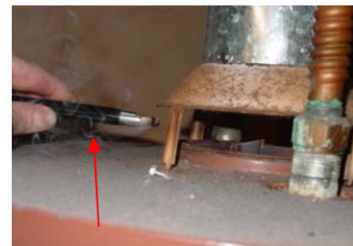
Figure 3122-2: Appliance fails spillage test
