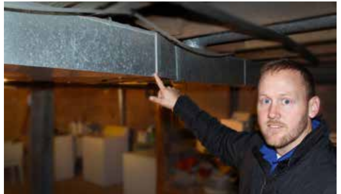
WCMCA auditor Gene Wyttenback pointed to the sealed duct work in the basement.
