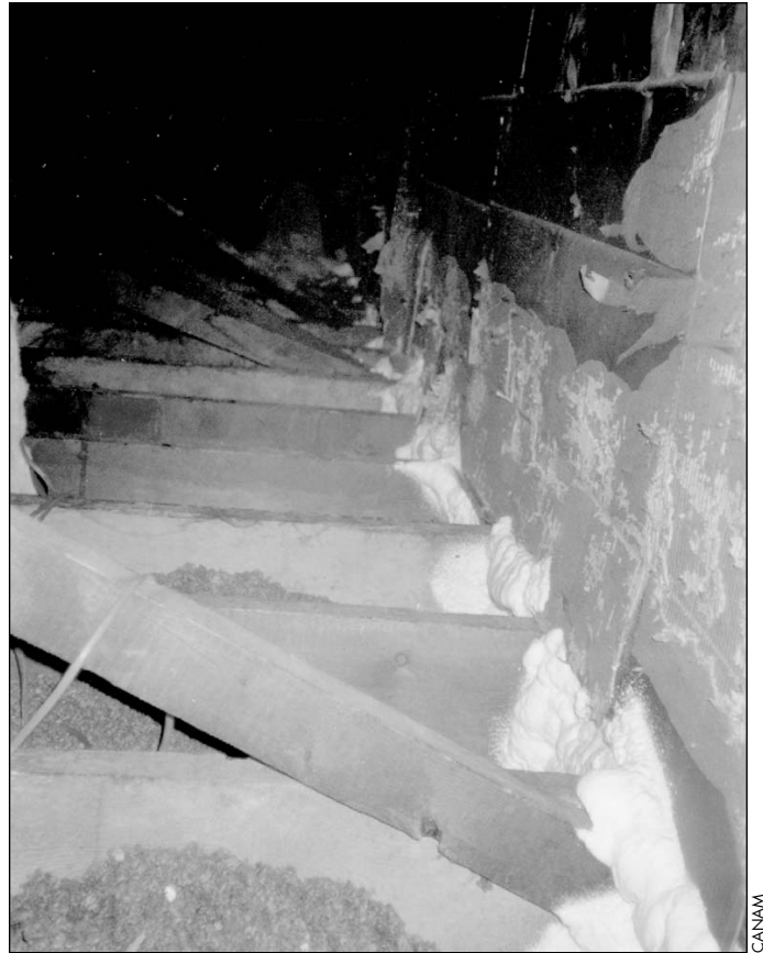
For kneewalls, the top plates and the joist cavities under the half-story are sealed with foam.
