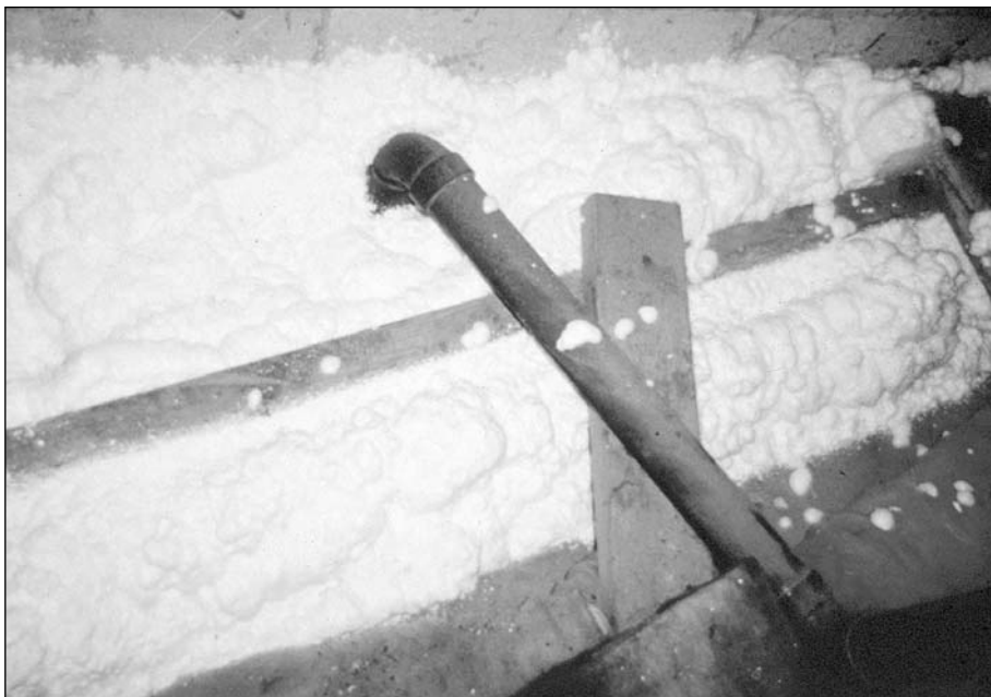
This hole between the attic and the party wall needs to be stuffed with mineral wool and then foamed.
