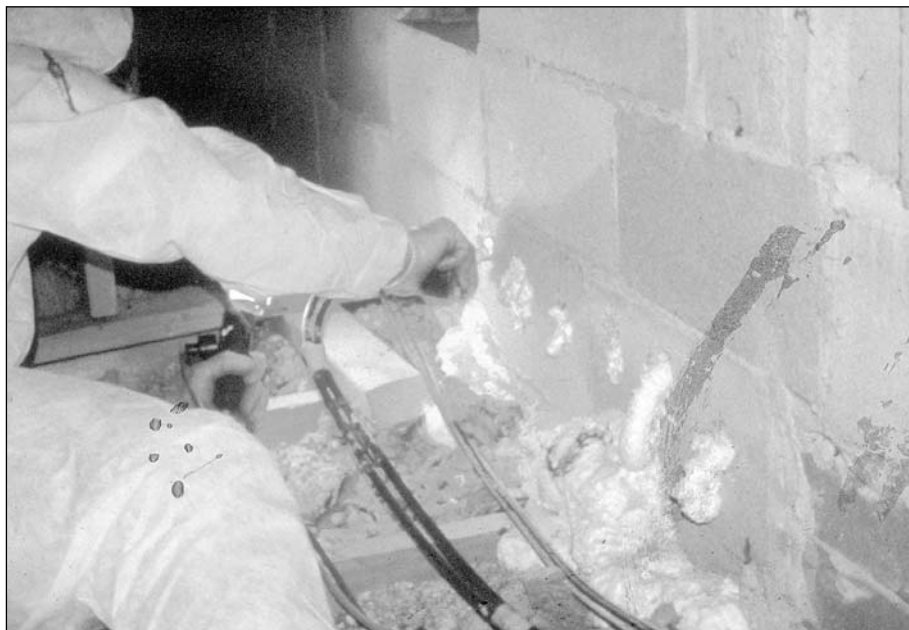
The crew always wear complete safety gear, including a disposable Tyvek suit. Here, one crew member is foaming into block cores to stop stack effect within the party wall.
