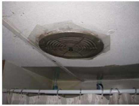
Completely non-functional bath fan.
