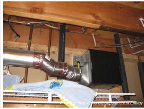
Brand new installation of a bath fan.
