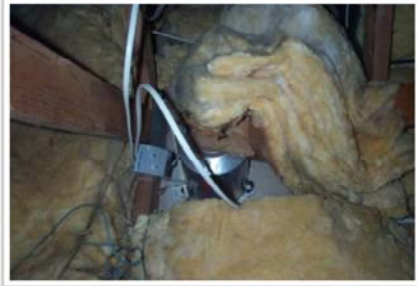
Leaky recessed lighting fixtures...
