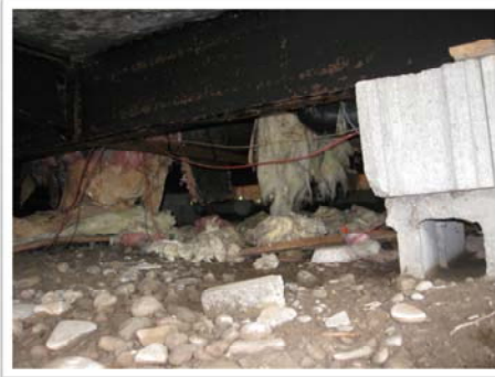
Collapsed insulation on a mobile home belly left untreated.
