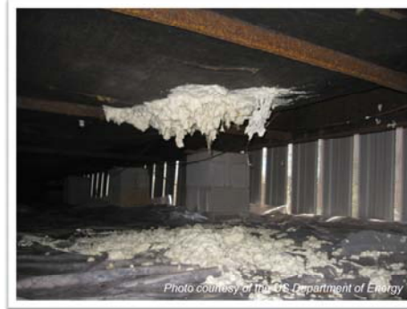
Mobile home belly penetration sealed but poor quality workmanship.
