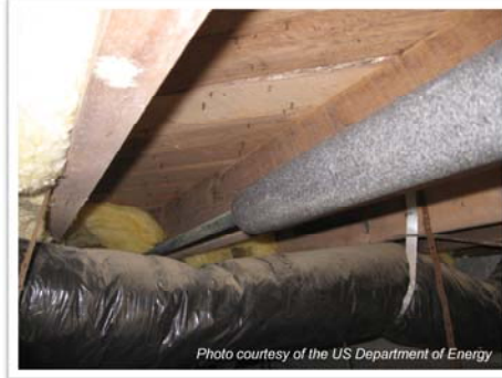
Missing floor insulation.
