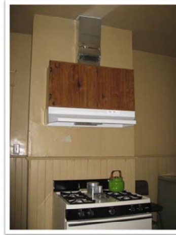
New range hood fan vented to outside.
