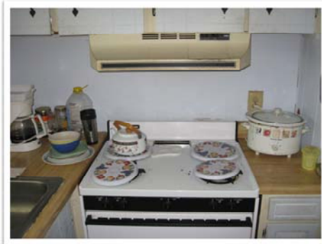
Unvented range hood over a gas cook stove.
