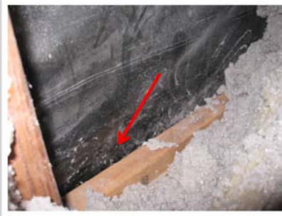
Entire length of top of marriage wall in a modular home was left unsealed prior to insulating attic.
