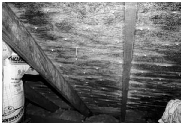
Saturated, warped and molded roof sheathing is often a result of warm, moist house air coming into contact with cold roof surfaces.
