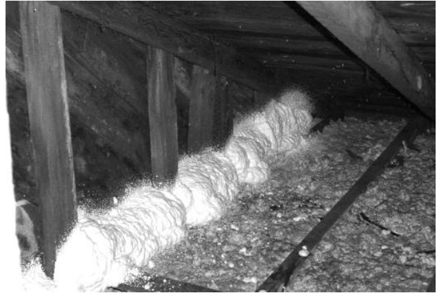
Fiberglass backer material stuffed into attic bypasses and encapsulated with triple expanding two-part foam creates a very fast and effective air barrier. In this case the installer applied a lot more than necessary to get the job done.
