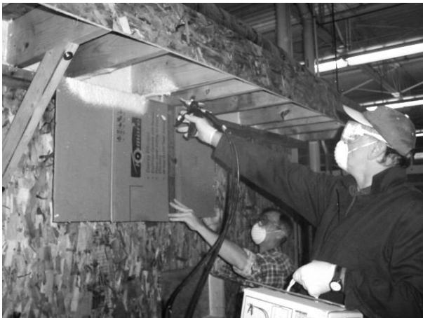
Two-part foam is being applied to a band joist mock-up using a wide spray pattern tip. The operator should be within six to twelve inches of the target area to prevent waste and overspray.
