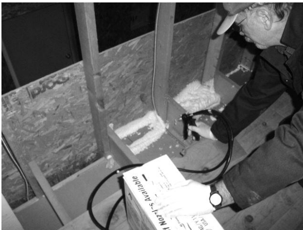
Two-Part Foam is being applied to open topped stud bays. The installer should be wearing a NIOSH approved breathing respirator.
