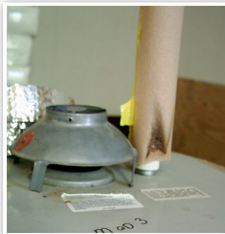
Insulating pipes too close to burner can be hazardous.
