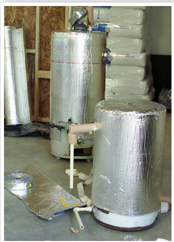
Wrapped water heaters. Leave 3" exposed at bottom to detect leakage. Don't cover top of gas water heater.
