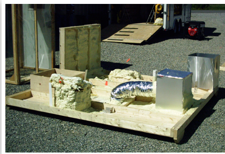
The finished prop with sealed and insulated ducts and a continuous air barrier.
