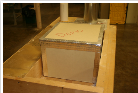
Detail of can light cover. Requires skill in measuring, cutting, and fitting.
