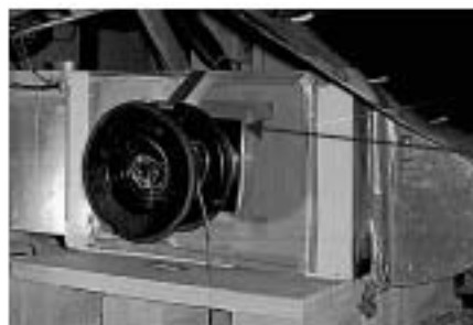
Main return is disconnected and the air handler is sealed.
