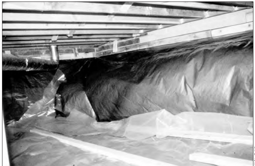
A well-sealed membrane installed in a crawlspace in Spokane, Washington, filled with soil air drawn from the highly permeable soil and by natural house depressurization. Exhausting air beneath the membrane solved this problem.
