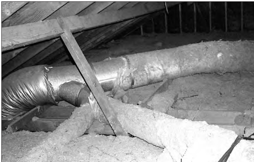
Here we see the poorly insulated sheet metal ducts and blown-in insulation in the attic before the retrofit.
