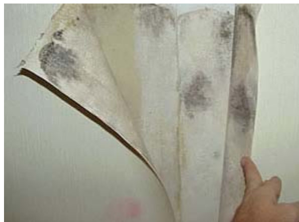
Note the pink "splotch" at the bottom-center of this photo. It is the telltale warning sign that there is a likely mold "bloom" behind the vinyl wall covering.
