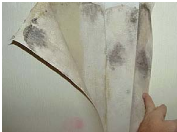
Note the pink "splotch" at the bottom-center of this photo. It is the telltale warning sign that there is a likely mold "bloom" behind the vinyl wall covering.
