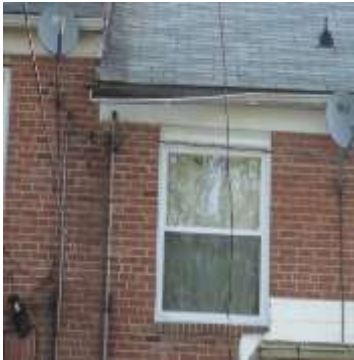
Defective gutters causing water leaks
