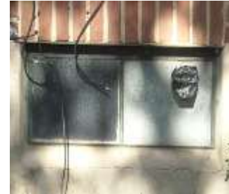
Deteriorated inefficient windows
