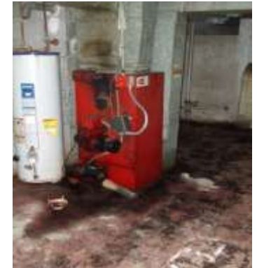
Broken hot water heater and furnace
