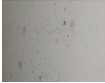
Water leaks creating mold hazards
