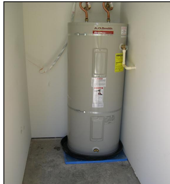
Hot water heater, drip pan, insulated under
