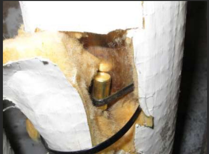
Exposed heating supply and return sensors
