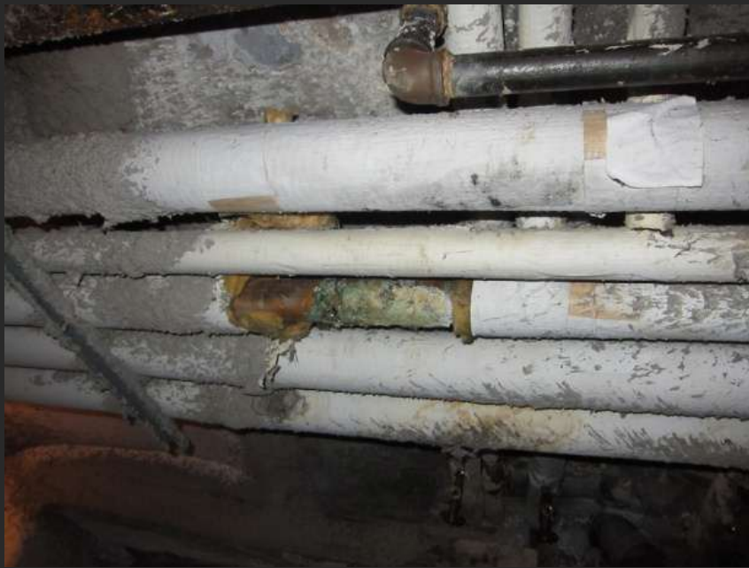
Missing & corroded insulation in distribution piping
