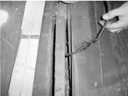
After removing a section of tongue and groove flooring in the attic, a taped splice was found. This splice was made in two pieces of rubber extension cord supplying power to a kitchen fan/light combo
