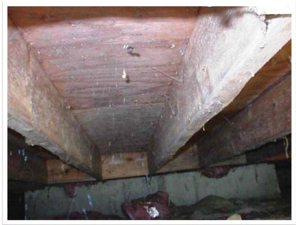
Mold growing on floor stringers over a dirt-floored crawl space.
